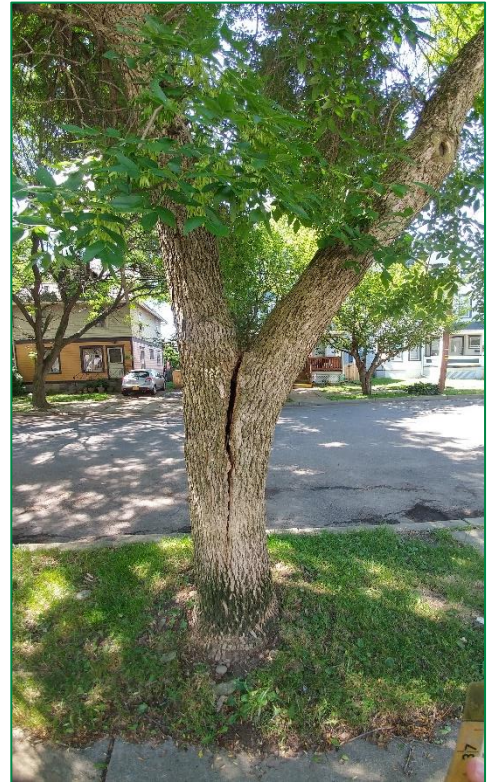
Photograph 2. The green ash (Fraxinus pennsylvanica) located at 6 Lawton Avenue has poor structure. With the location of the tree, size of defect, and potential for failure, this tree was assigned a High-Risk rating. Given the severity of the split crotch, as well as the species consideration, Removal is recommended.
