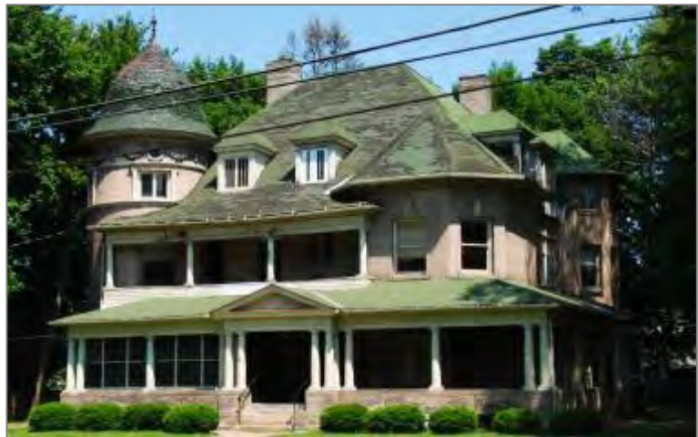
The roof of this Queen Anne structure is in need of repair and general maintenance and upkeep. The water damage is an example of a problem that can arise as a result of deferred maintenance.
