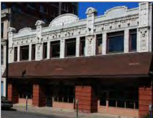
The integrity of the Strand Theatre has been compromised by inappropriate treatments on its historic façade.
