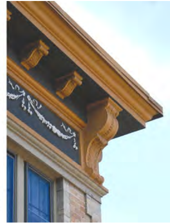
The cornice of this Neo-Classical storefront is historically intact due to good maintenance.
