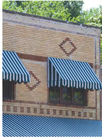
The visual border cornice of this 1920s storefront has been compromised by an inappropriate repointing job.
