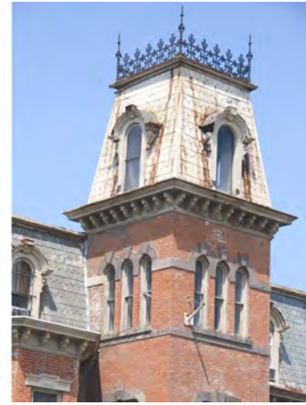
Rust staining is evident on the roof of this structure, resulting from deferred maintenance of its metal roof features.
