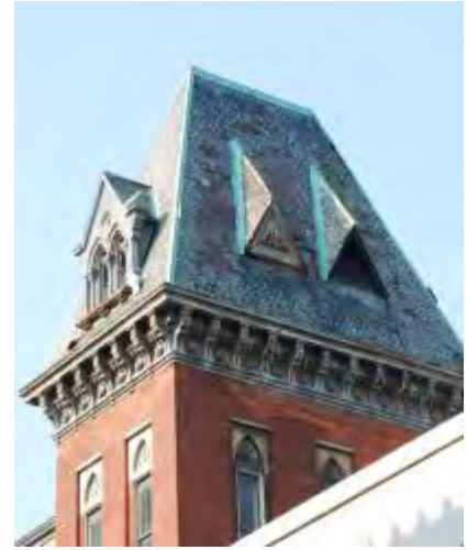
The deterioration of the roof and gutters of this building has caused roof elements to have significant corrosion issues in addition to water damage to the brick wall below.
