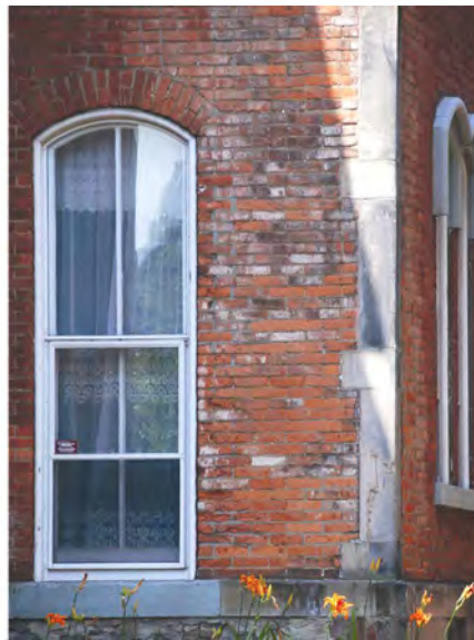
The bricks of this building have begun to spall significantly because of inappropriate cleaning methods and exposure of the originally painted brick.
