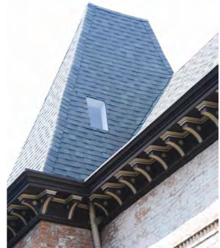
While the cornice of the building has been restored, the integrity of its roof has been compromised through the improperly installed skylight, asphalt shingles, and removal of its roof ridging.
