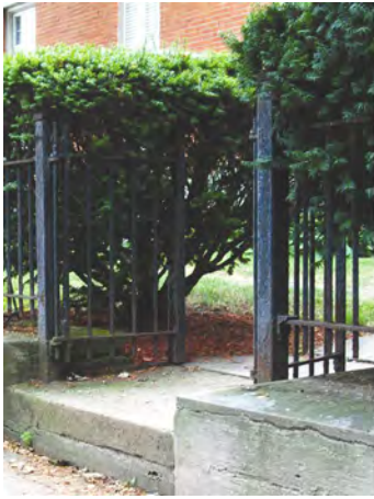
This iron gate and fence has deteriorated, as evidenced by rusting, from lack of proper painting maintenance.
