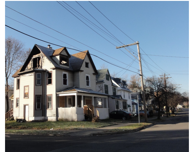
Vacant and distressed properties can be assembled through the County Land Bank.
