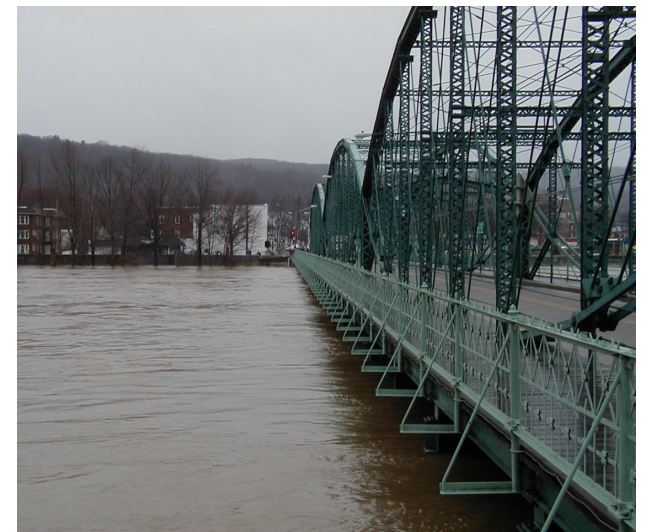
Flood Waters at the Washington Street Bridge
