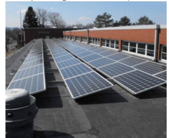
Solar Array on the Binghamton Water filtration plant
