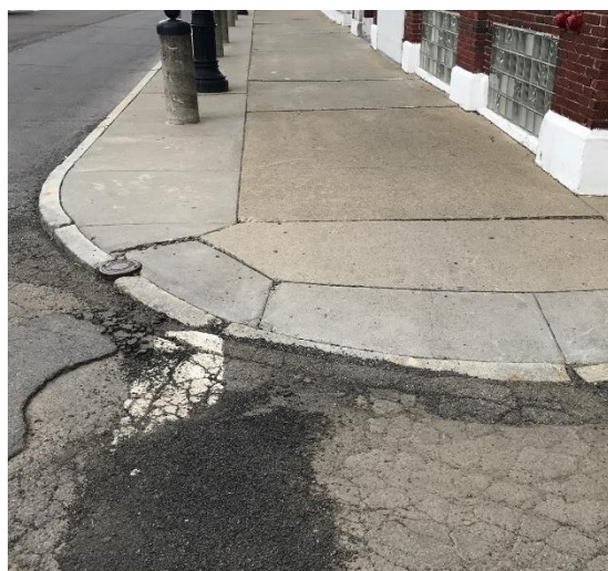
Example 3: No truncated domes are present; crosswalk painting is faded and covered in debris.
