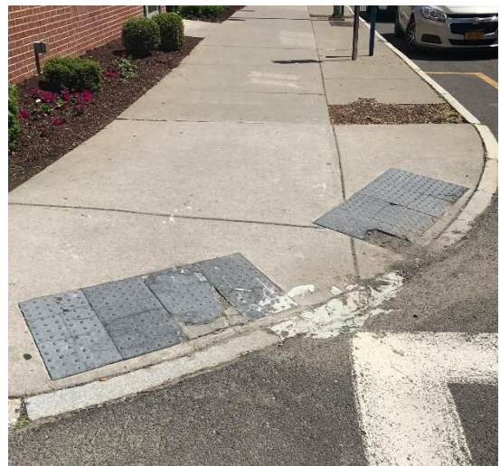
Example 4: While truncated domes are present on the curb ramps, they are old and deteriorated.
