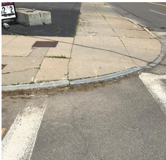
Example 1: Curb does not come flush with the road; sidewalks are uneven.
