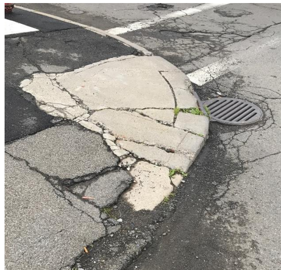
Example 2: Sidewalk and curb ramps are very uneven and crumbling; only one crosswalk is present.
