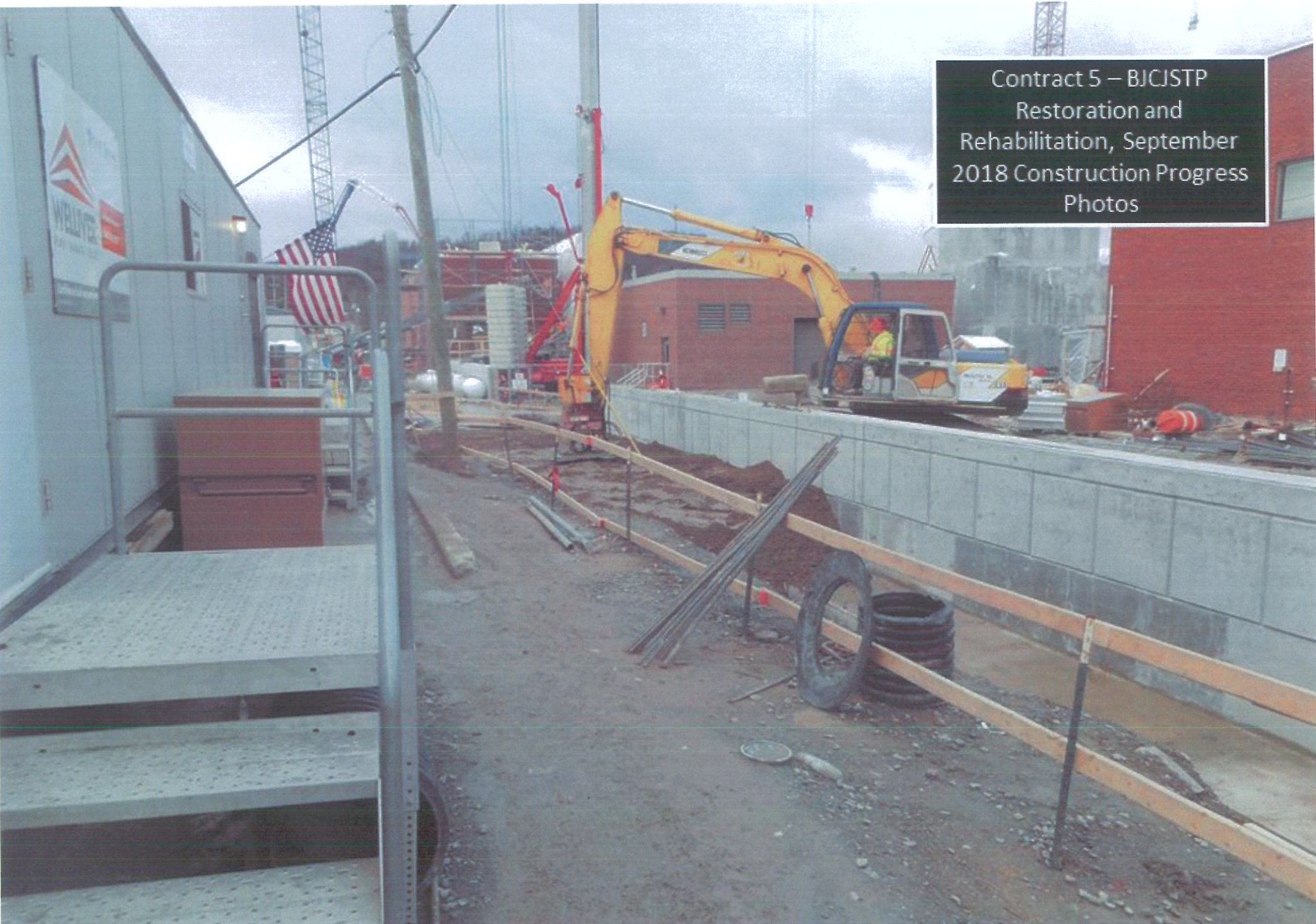
South Flood Wall - Back Filling Around the Flood Wall Extension South of the Generator Building
