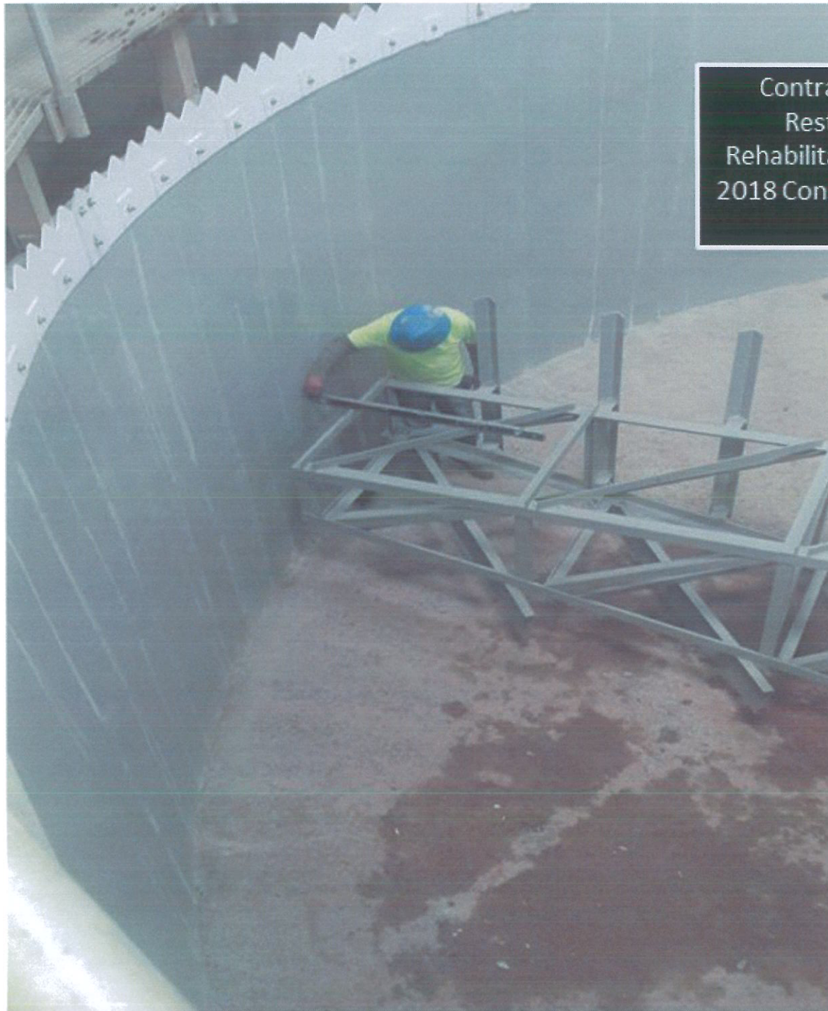
Sludge Thickener No. 1 – Leveling Rake Arms
