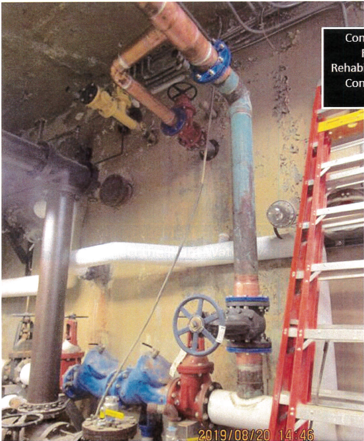
Digester Control Building Basement – Field Work Directive Work to Reconnect the Plant Water System
