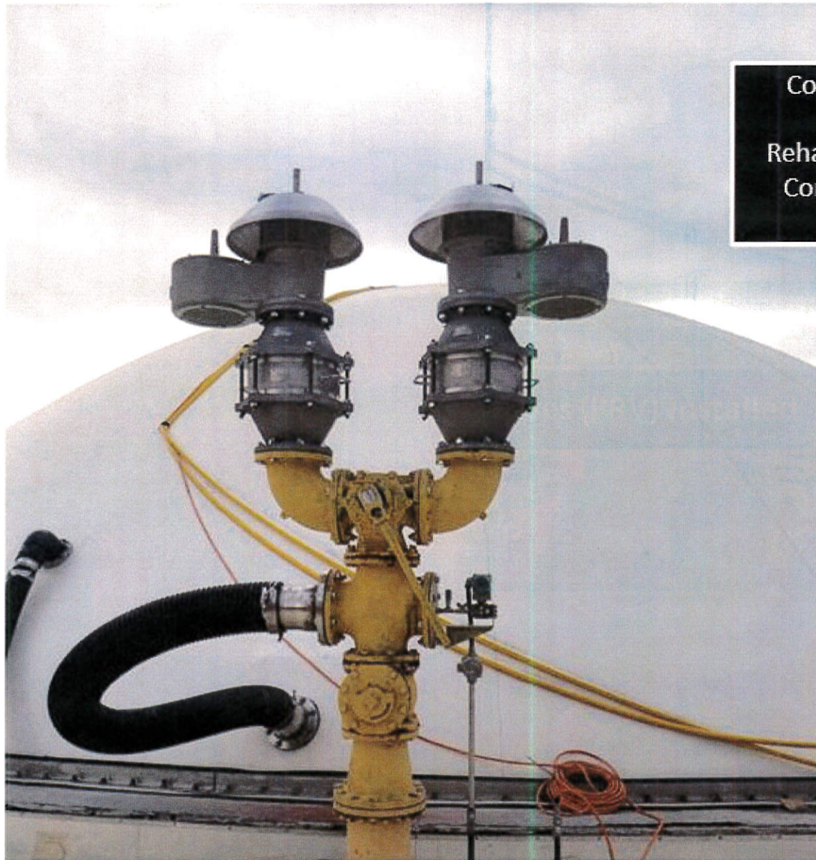
Digester Tank 3 – Pressure Relief Valves (PRV) Installed
