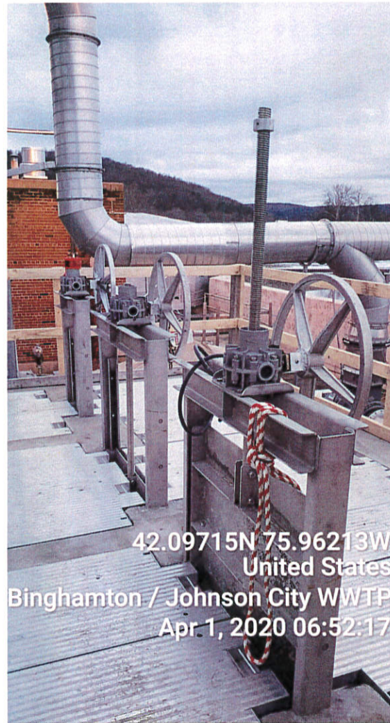
Sludge Thickener Distribution Box Online
